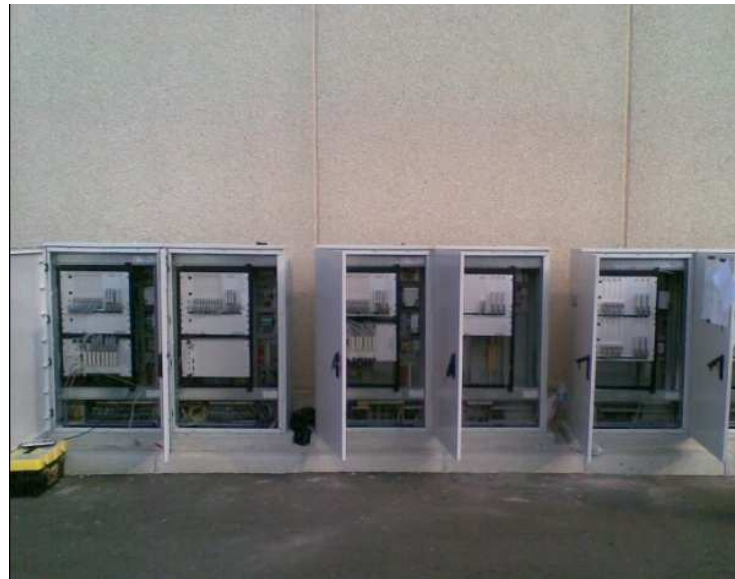
Signalling Cabinet For Depot Application
